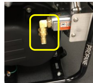
Propane & natural gas inlet location. Note protective cap removed for access
